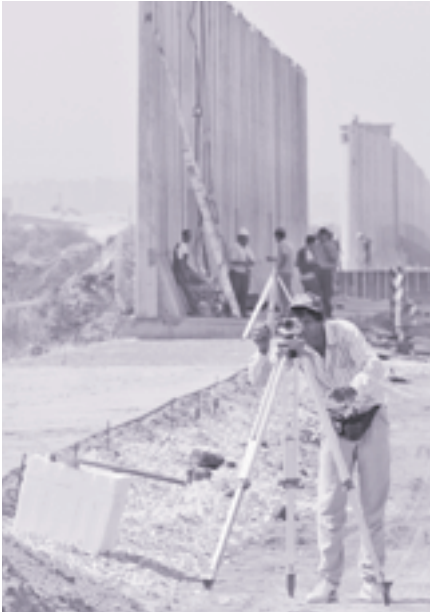
The early beginnings of the fence being built along the Green Line, separating Israel from the West Bank. This part of the fence is near the Israeli town of Kfar Saba. July 2002.
