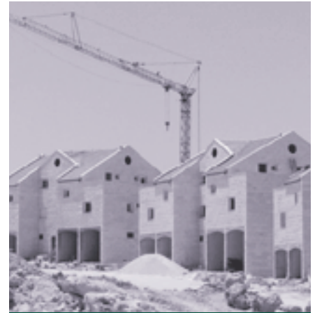
Construction of new homes in the West Bank settlement of Efrat. May 2001.
