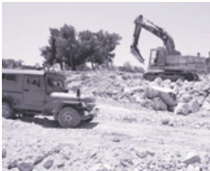
Construction is being done to prepare the ground for an electronic security fence between Bethlehem and southern Jerusalem. The fence will stretch 50 km. (30 miles) and surround Jerusalem on three sides. July 2002.
